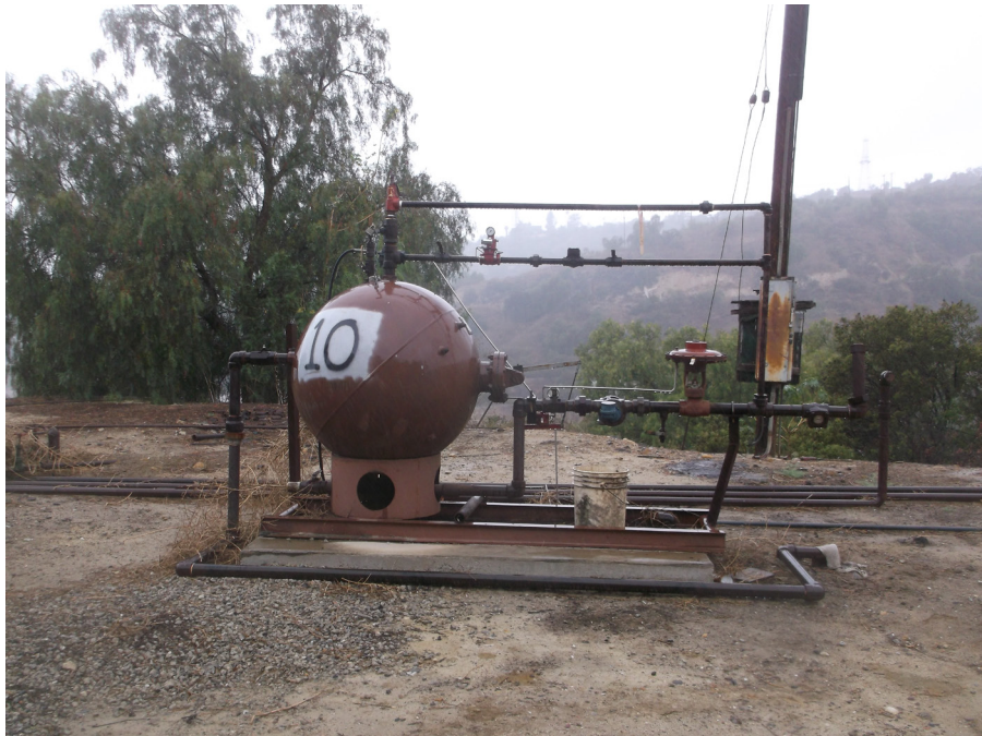
Plate 23: Brea Well #71 Oil and Gas Separator, View North.
