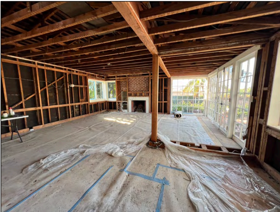
Photo 26. Main dwelling, interior view of header beam at the original north-facing exterior wall location.
