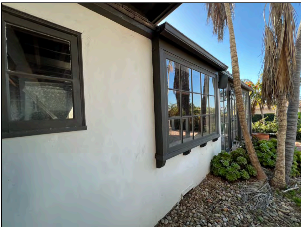
Photo 24. Main dwelling, north-facing facade with window installed out from wall plan (center) and altered wall / enclosed porch (center and at right).
