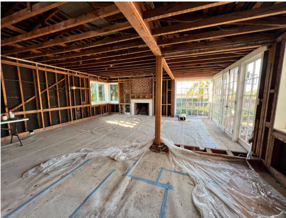
Photo 26. Main dwelling, interior view of header beam at the original north-facing exterior wall location.
