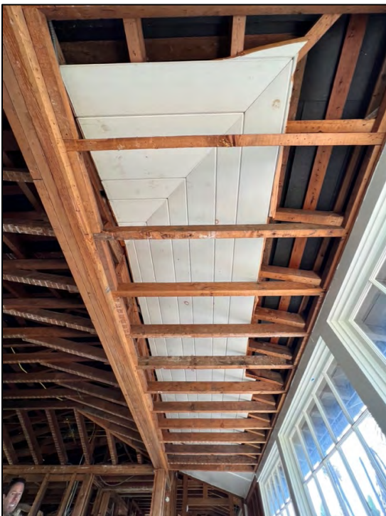
Photo 28. Main dwelling, interior view of original 2nd level porch / balcony enclosed with original soffit boards exposed above new framing.
