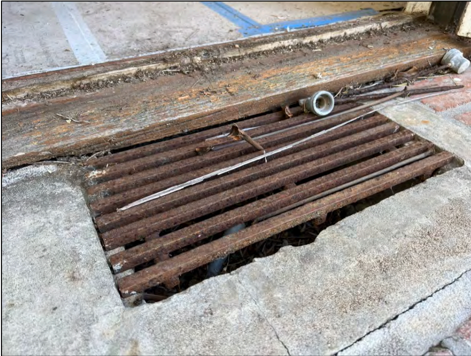
Photo 29. Drainage grate installed. Several grates are installed around the main dwelling footprint to prevent water infiltration.
