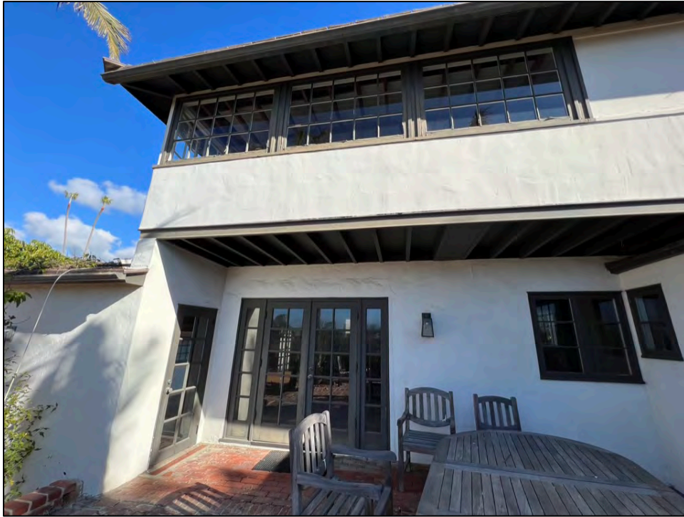
Photo 21. Main dwelling, west elevation fenestration at west-facing facades with non-original French doors, and inelegant placement of wood windows at the west-and-north-facing wall junction (at right).
