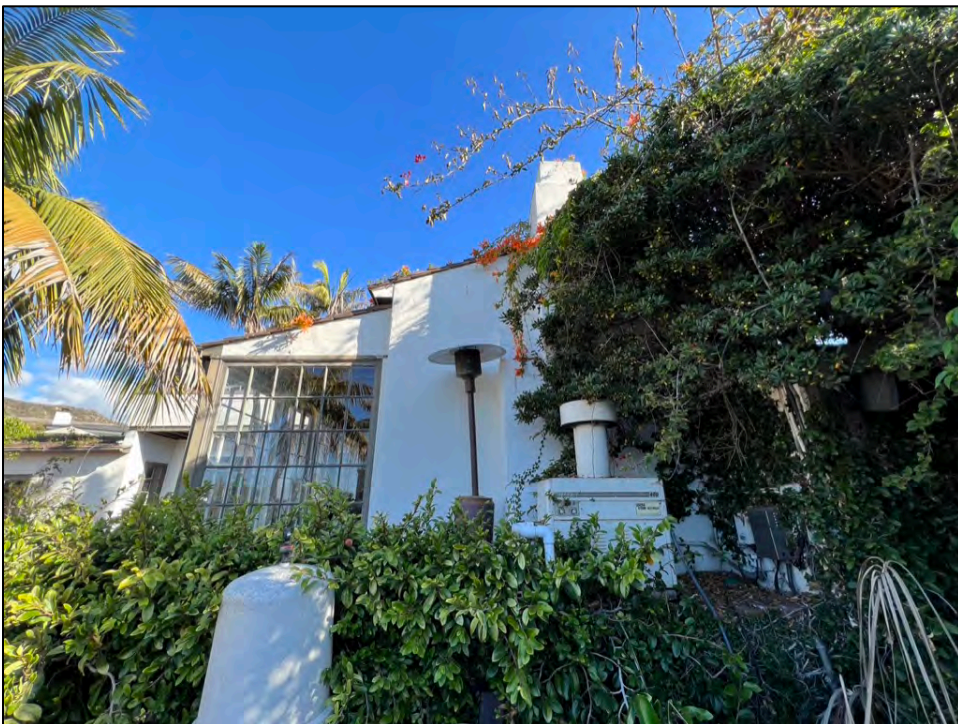
Photo 18. Main dwelling, west elevation showing altered / enclosed north-facing wall within the single-story wing.
