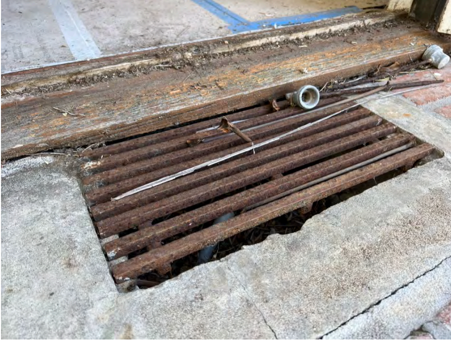
Photo 29. Drainage grate installed. Several grates are installed around the main dwelling footprint to prevent water infiltration.
