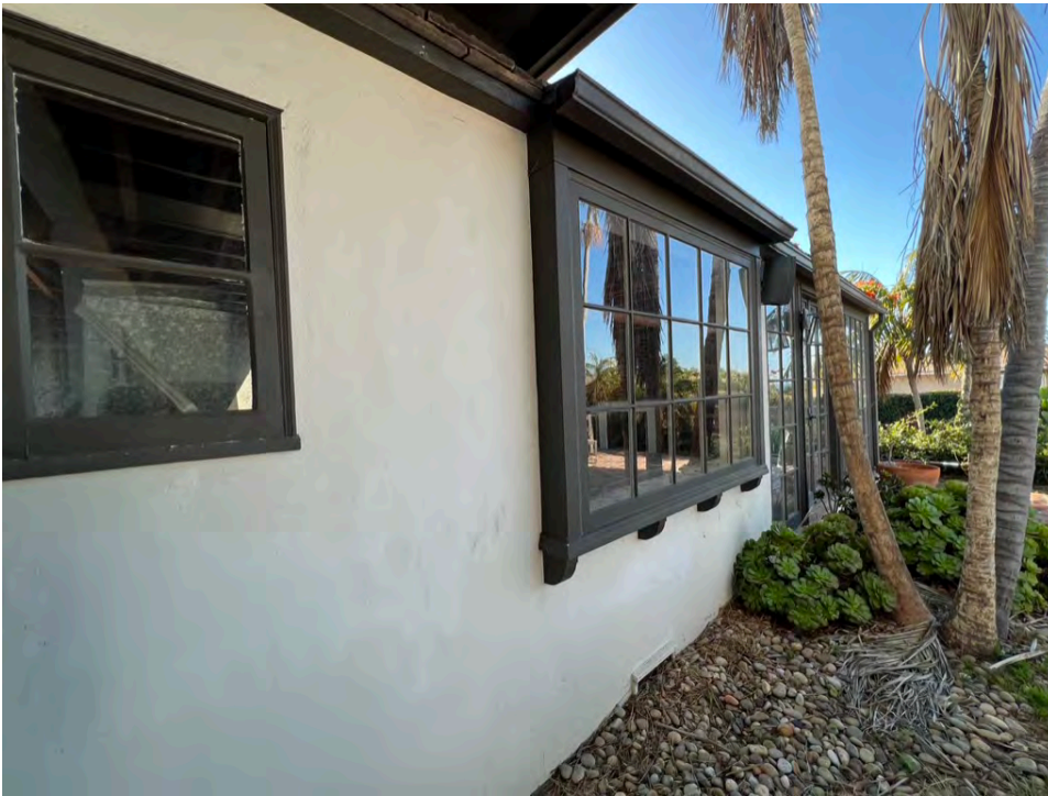
Photo 24. Main dwelling, north-facing facade with window installed out from wall plan (center) and altered wall / enclosed porch (center and at right).
