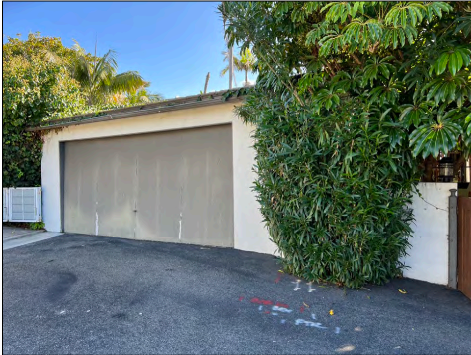
Photo 33. North lot line, north elevation of detached garage, sited east of the courtyard gate.
