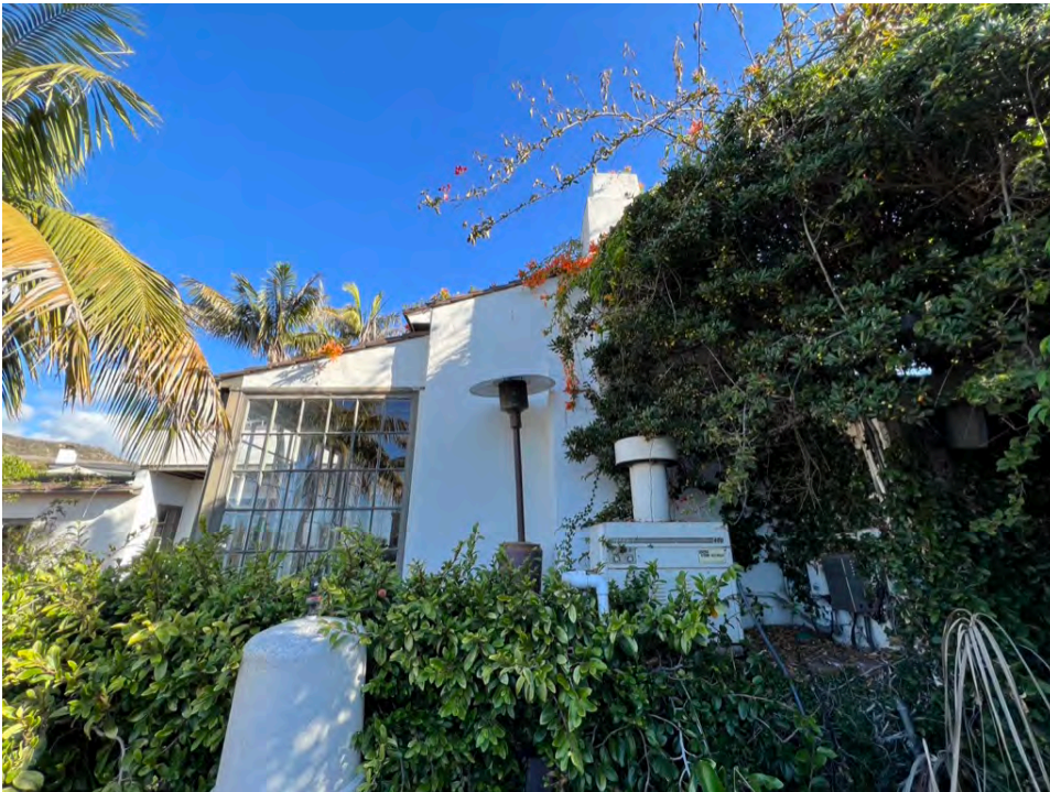
Photo 18. Main dwelling, west elevation showing altered / enclosed north-facing wall within the single-story wing.
