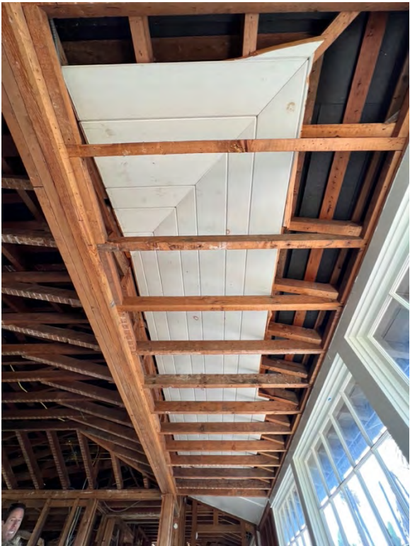
Photo 28. Main dwelling, interior view of original 2nd level porch / balcony enclosed with original soffit boards exposed above new framing.
