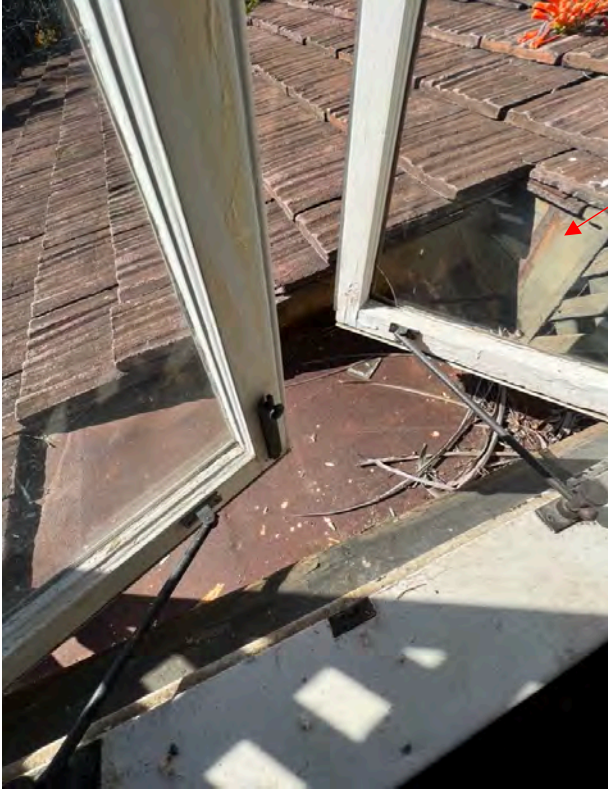
Photo 3. View of covered shaft / gap between the two-story volume and the single-story wing. Lattice is extant at the north side of the opening, indicating a balcony may have been removed.
