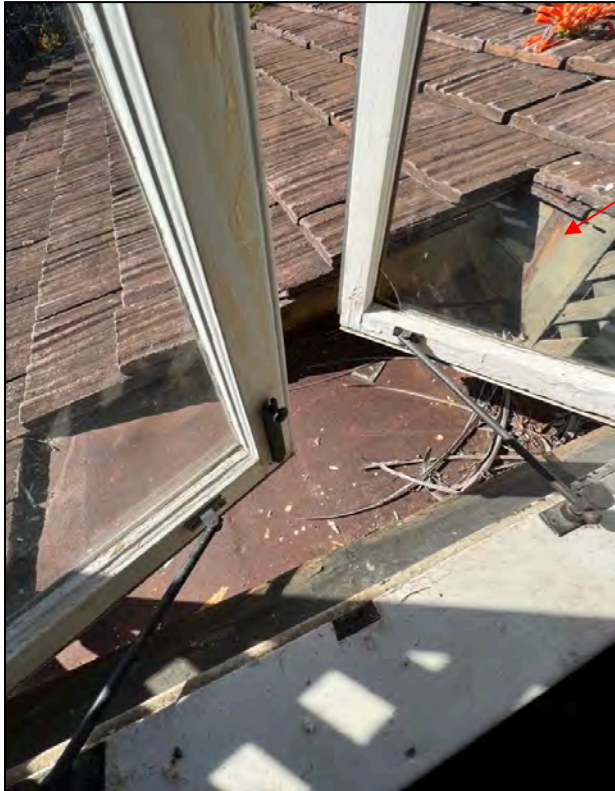
Photo 3. View of covered shaft / gap between the two-story volume and the single-story wing. Lattice is extant at the north side of the opening, indicating a balcony may have been removed.
