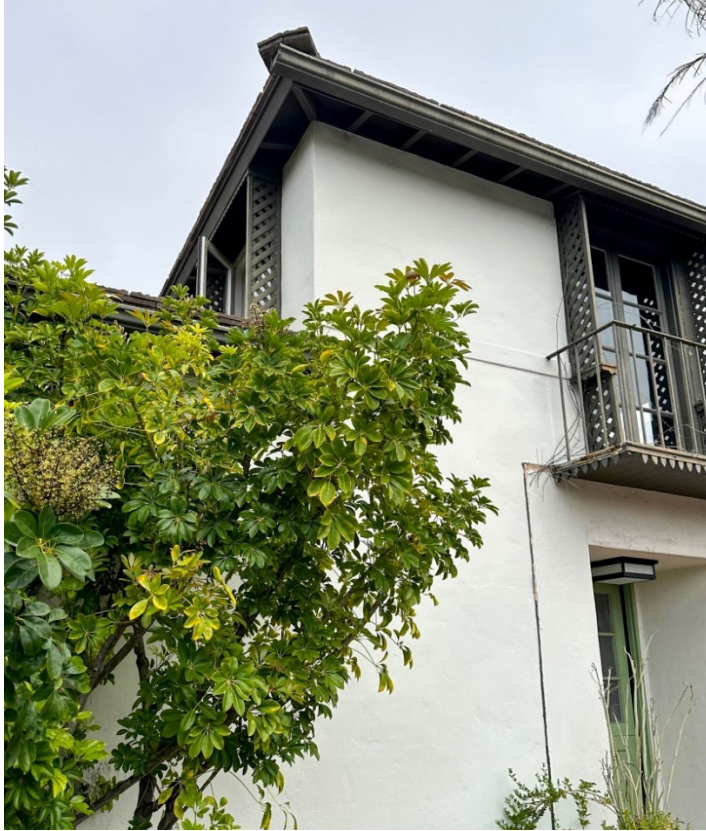
Figure 3. Details of overhanging roof eaves and wood lattice around the windows. South elevation, view looking northeast. Source: ESA 2023.
