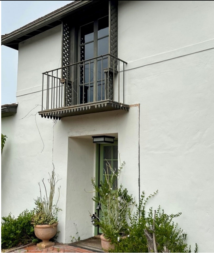
Figure 2. Detail of the stucco and original wood ornamental design around the entrance. The wooden lattice under the balconette that surrounded the entrance has been removed. South elevation, view looking northwest. Source: ESA 2023.
