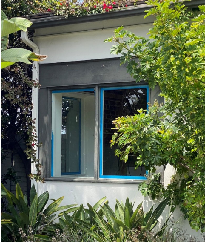
Figure 6. Detail of a non-original window on the south elevation, view looking north. Source: ESA 2023.
