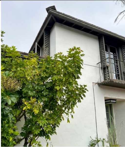
Photo 5- Detail of overhanging roof eaves and wood lattice frame around the second story windows on the northwest elevation. Northwest and southeast elevation, view looking northeast. Source: ESA 2023.
