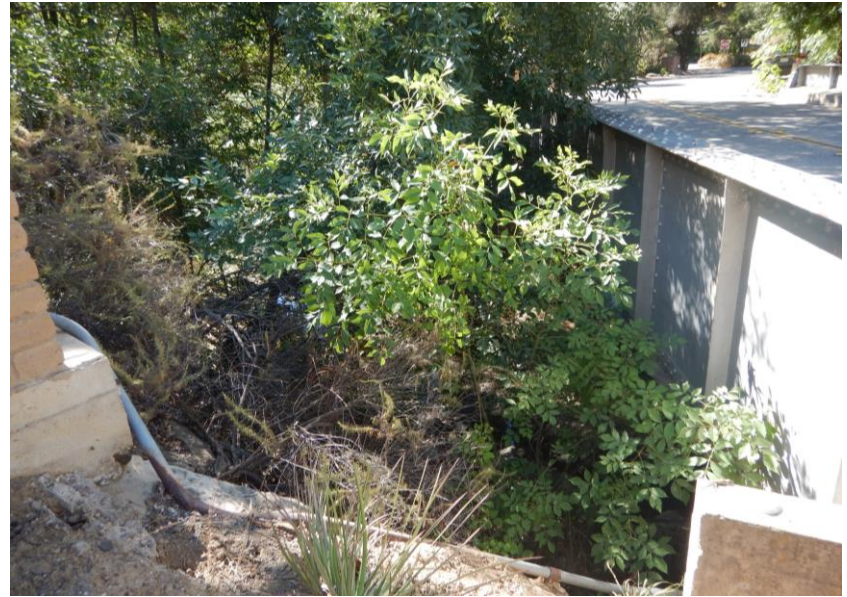
Photograph 4: View looking south from Modjeska Canyon Road/Markuson at Santiago Creek. Latitude 33.708843°, Longitude -117.636358°.
