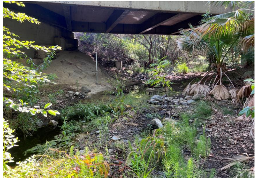
Photograph 2: View looking east at the Modjeska Grade Road Bridge spanning Santiago Creek. Latitude 33.708703°, Longitude -117.636444°.
