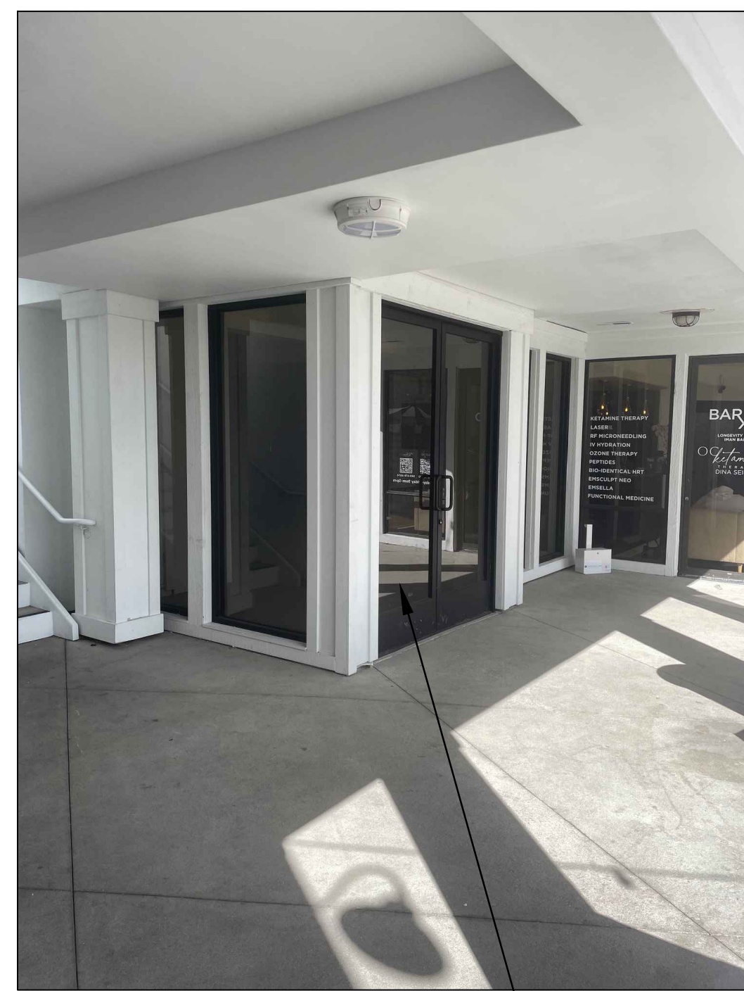
LOUNGE BAR SUITE D1 DOOR AT FIRST FLOOR
