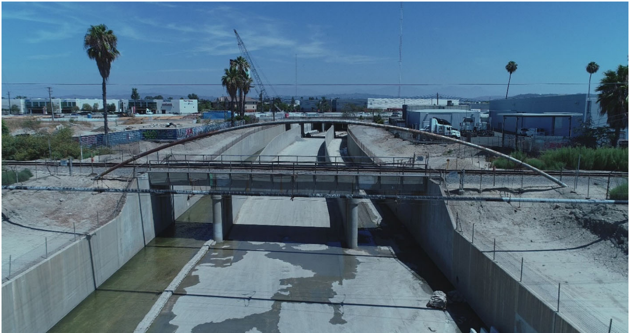
UPRR Industry Lead over Coyote Creek (looking upstream from downstream of bridge)
