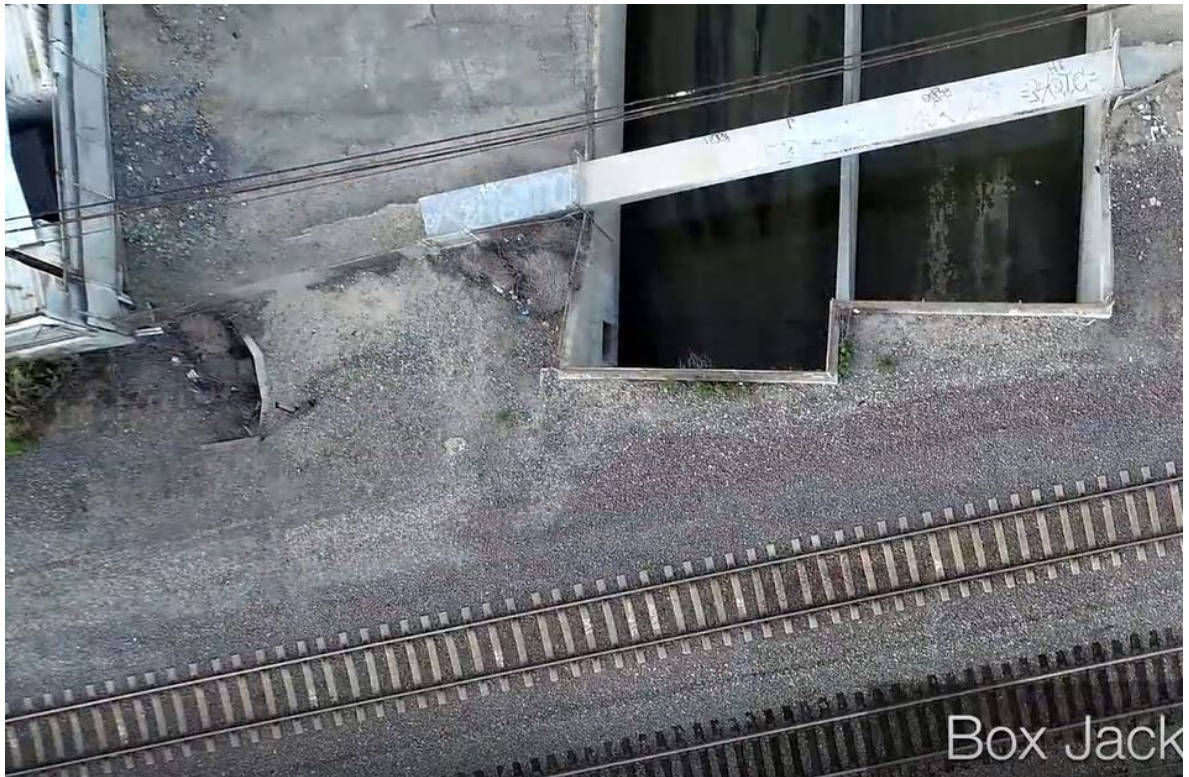
Existing 36" Side Drain and AT&T Duct Bank (in concrete box girder) Upstream side of BNSF/Metrolink Bridge over Coyote Creek
