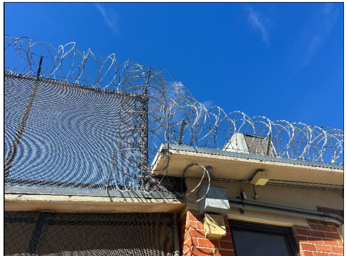
Building #5, character-defining materials: chain link fence, coiled razor wire at the junction of the cast-in-place concrete roof and exterior brick wall (10/21/24).
