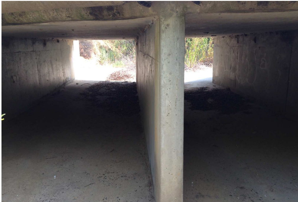
Photograph 12: Long north in Drainage C beneath Long Canyon Road. Flows from drainage are conveyed within two box culverts.
